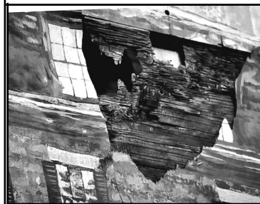
Bricks showing thru where paint is torn off from weather.
